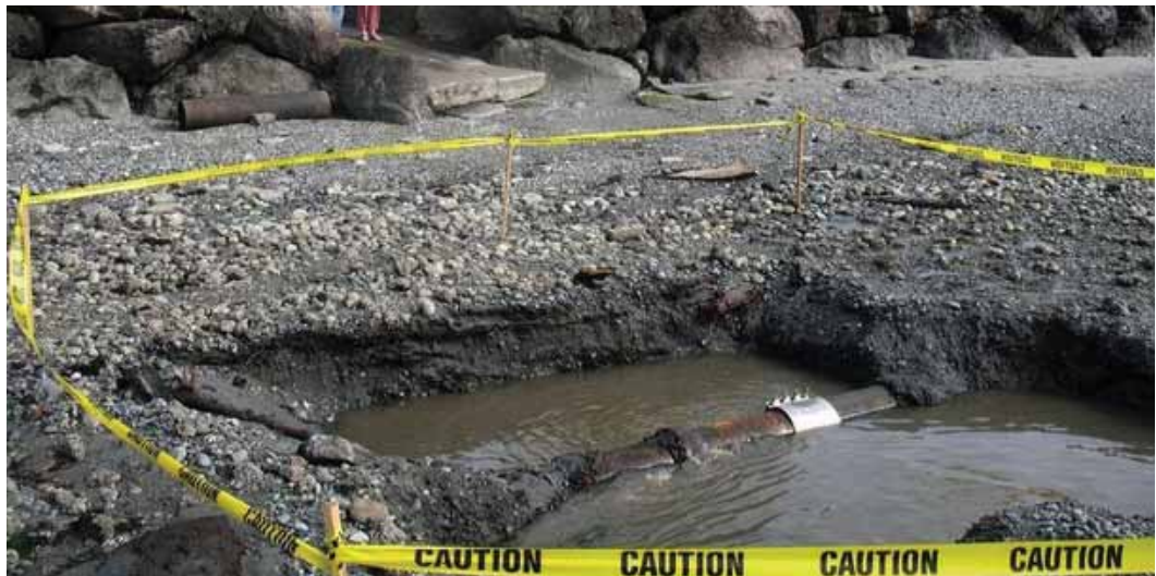
Sewage pipe leak at Eagle Harbor, Bainbridge Island, June 2009.
